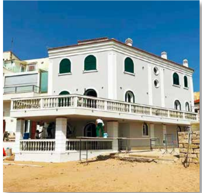
RAGUSA: Building used as the set for a famous Italian TV series "Il Commissario Montalbano". Facade treated with AFONTERMO®
